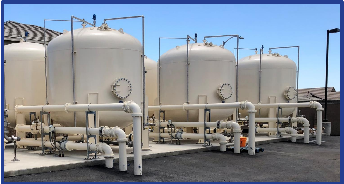
TCP Treatment Facilities recently constructed at City of Livingston Well 16.
